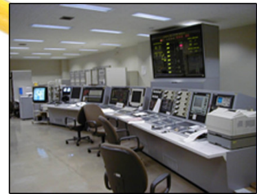
Process control system
